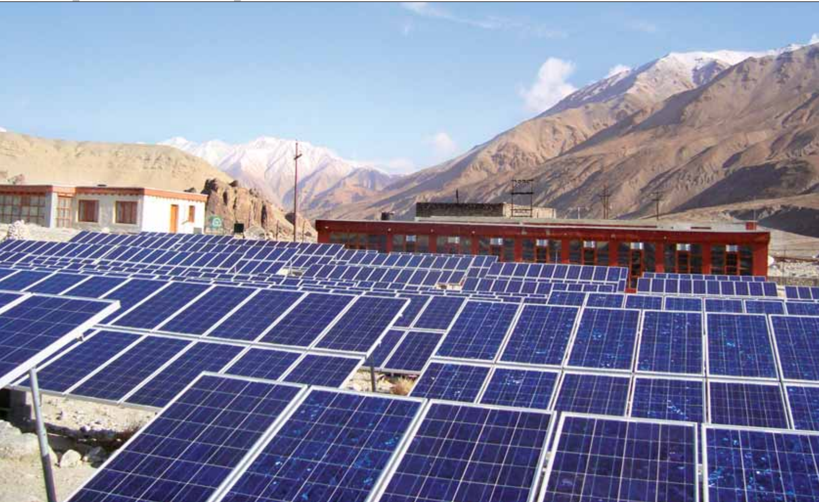
100 kW Tangtse Solar Power Plant, Ladakh
